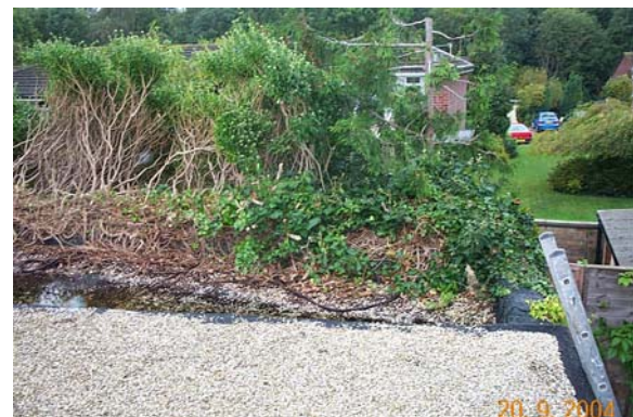
4. Extensive Ivy Growth on a Roof
